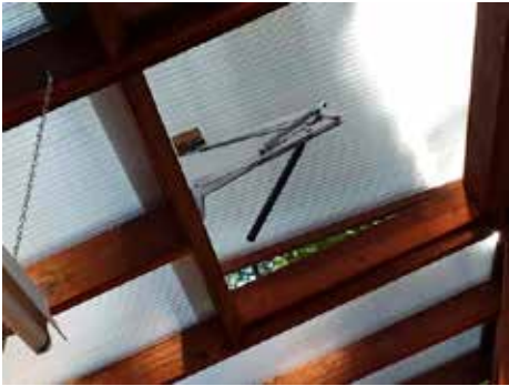
Roof vents are critical. They can be operated manually or with automatic openers. Photo by Bonnie Bradt
